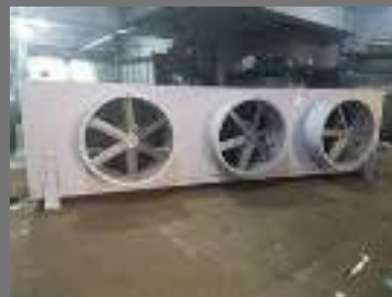
Ammonia air cooling unit for cold room
