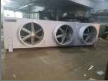
Ammonia Air Cooling Unit
