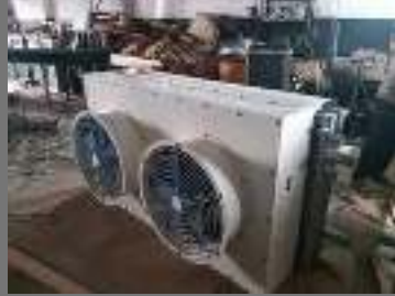
CNG Daughter Booster DRY COOLER
